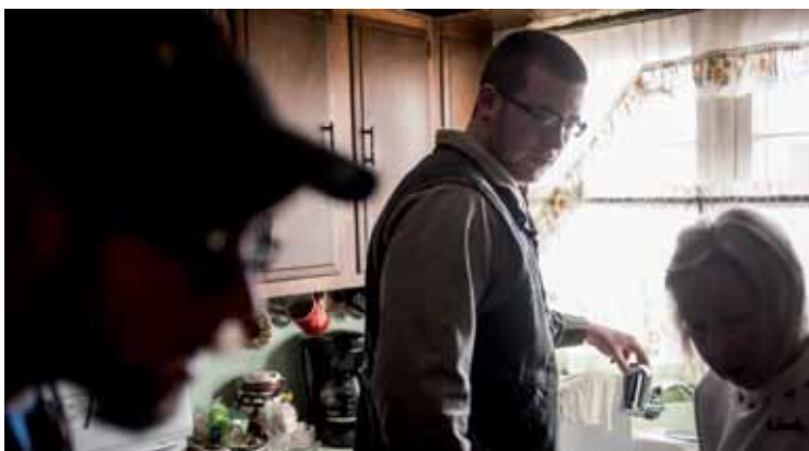
Plumbers installed state-provided filters in more than 1,500 homes around Flint, and new faucets in homes where existing products were not compatible.
